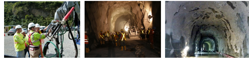
STI's experienced personnel worked with CNO's 700-men on site to deliver a successful job up to international standards
