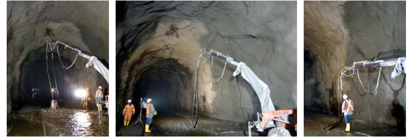
The combination of Shot-Tech Robotic Arms, Nozzles and Shot-Set 250 allowed for high quality shotcrete application
