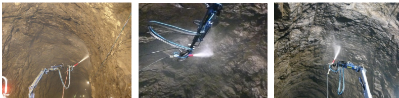
The Shot-Tech Arms and Nozzles played an unexpected role, when efficiently used to wash the upper part of the tunnel
